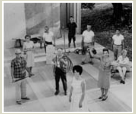
July 1963—Board members and volunteers finish work on the first stage. Bert Pree, Britt's first board president, is seated in the wheelbarrow.
